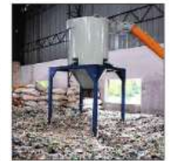
The ITC Limited facility for recycling MLP waste into plastic granules
